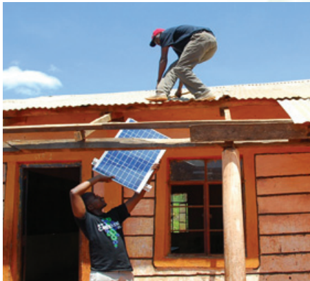
Kasiluni EPICS project lead, Gerald K. Too, from the IEEE Kenya Section hands over a solar panel during installation on the standard 6 classroom schoolhouse at Kasiluni Primary School in Northern Kenya.
