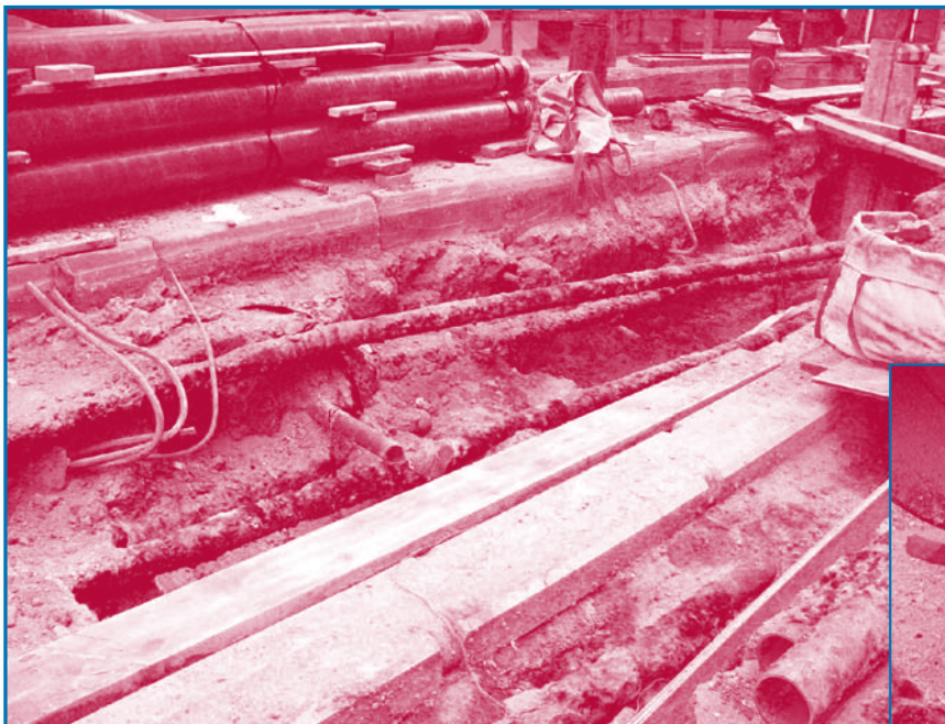
old Edison feeders suspended close to street
