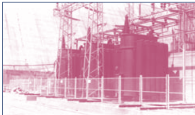
Transformers at Norris Dam Substation. Ellenberger collection photo
