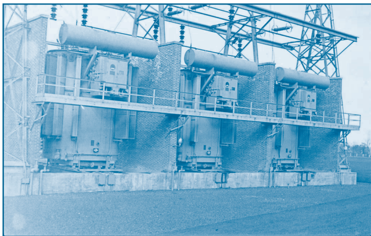
PSE&G's Roseland, New Jersey Switching Station
