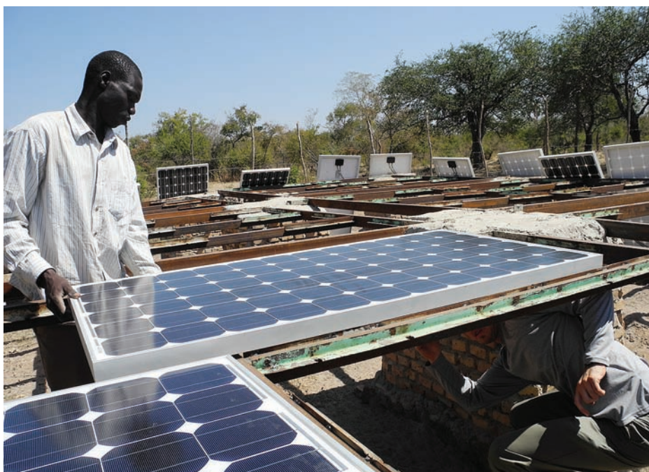
Entrepreneur Mou Riiny, a former refugee from war-torn South Sudan, returned to his village, Thiou, where he is installing 13 community charging stations powered by photovoltaic panels.
