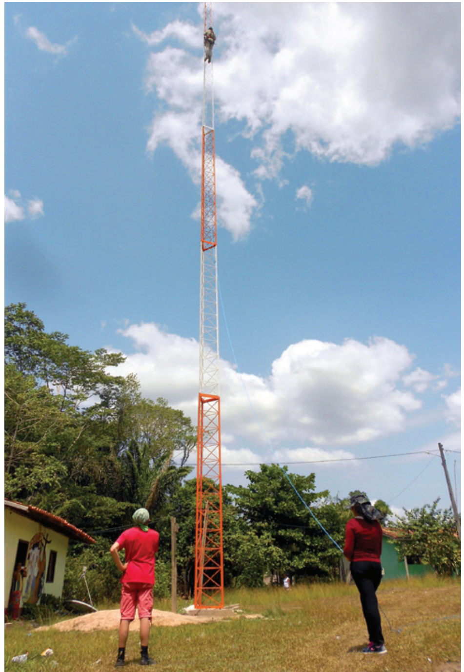
The new tower and base station enable cellular connectivity resulting in enhanced health, education and safety as well as the facilitation of small business development.
