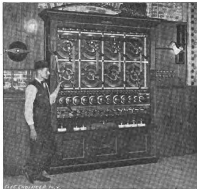
SWITCHBOARD, EMPIRE THEATRE, PHILADELPHIA.
