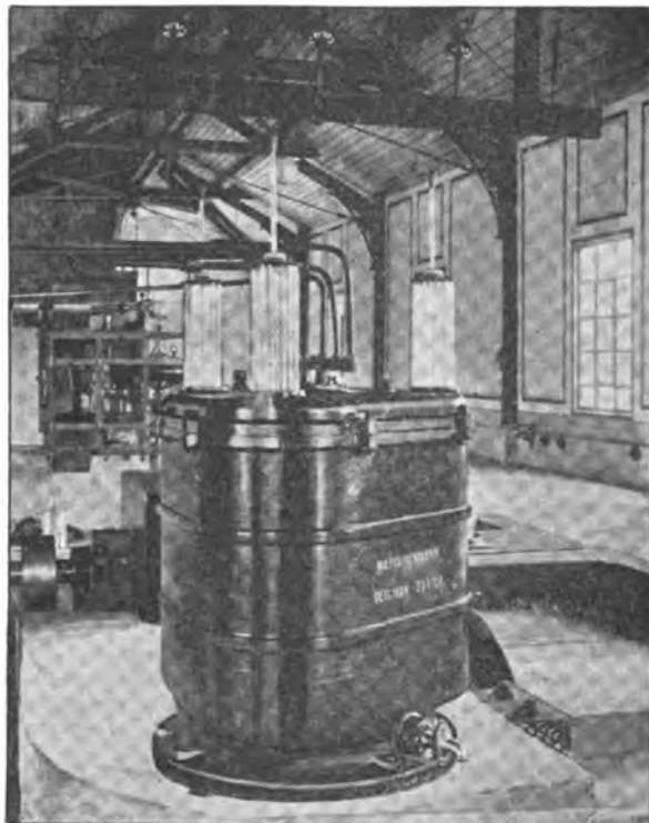
OERLIKON TRANSFORMER AT FRANKFORT.
