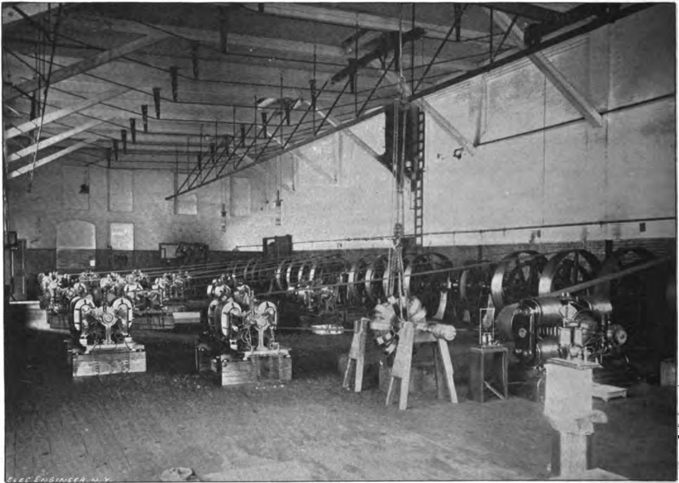
FIG. 2.—DYNAMO ROOM, BRUSH ELECTRIC LIGHT STATION NO. 2, BUFFALO, N. Y. (See page 279.)
