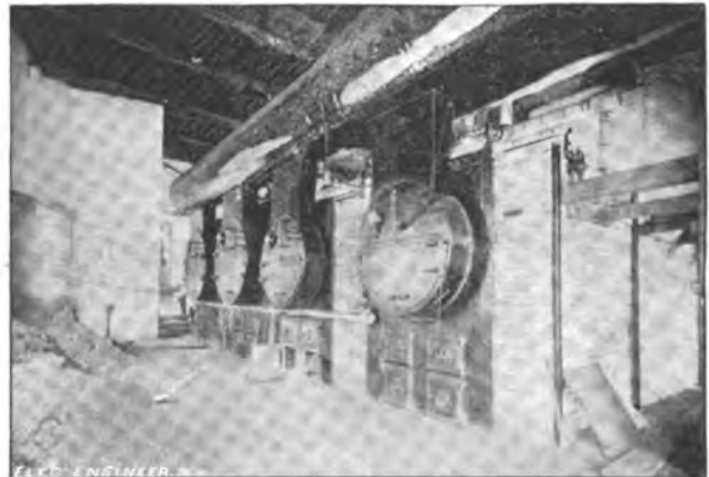
FIG. 4.—BOILERS, PITTSFIELD, MASS., ELECTRIC LIGHT STATION.
